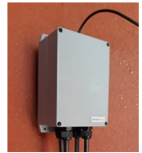
Figure 5 SENSECOM-HPC for measuring from up to 5 VW probes and sending data via IoT network
