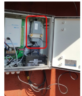
Figure 3 Meter panel with connection to SENSECOM-GL1 IoT communicator
